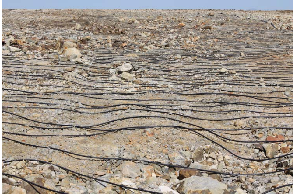
Figure 4: Part of the 4,000km dripper network on the site
